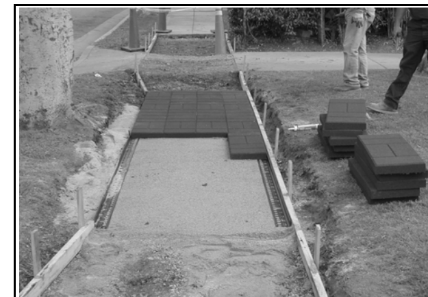
Installation of rubber sidewalks along the 2900 block of Delaware Avenue in the City of Santa Monica
