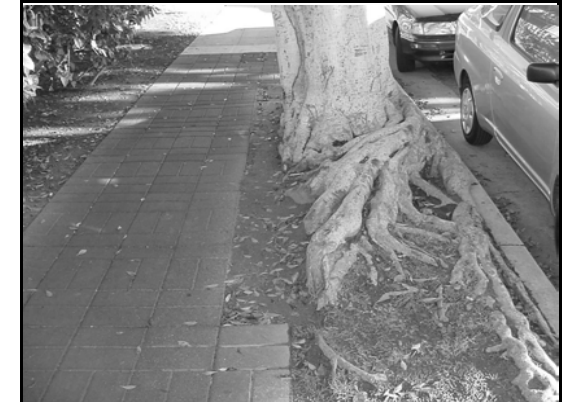
Santa Monica's first rubber sidewalk was installed in late 1999 at 21st Street and Ocean Park Blvd. Next to the Fairview Library.
